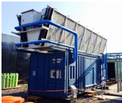
1 unit on CAT diesel
