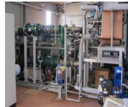
2 units on biomass boiler
